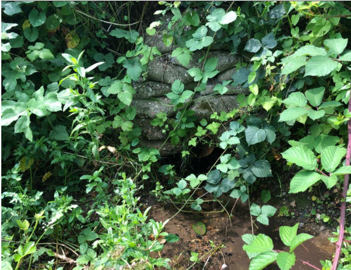
Plate 10: Outfall into Receiving Open Land Drain
