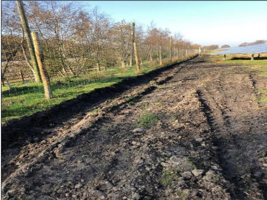
Plate 18: Example Perimeter Swale at a Solar Farm Site 33
